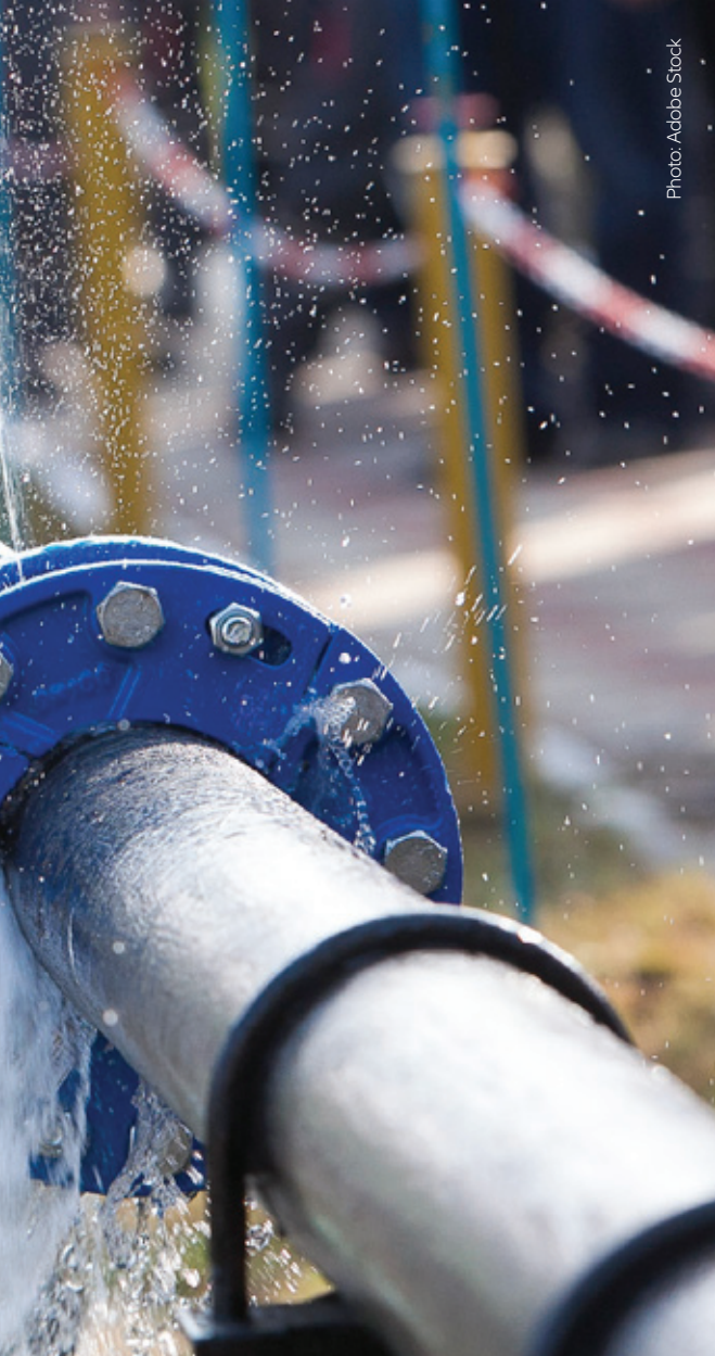
Damage to construction projects often occurs on weekends or holidays
