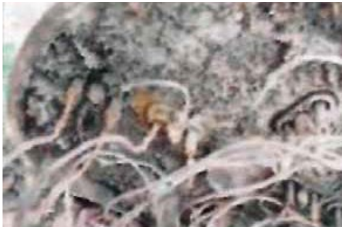
↑ The resistance-coil laden cover on the humidifier where the fire broke out
