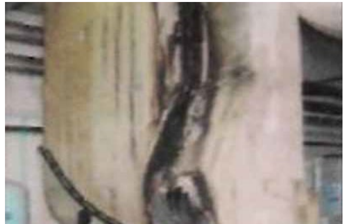
↑ The damaged humidifier and A/C casing
