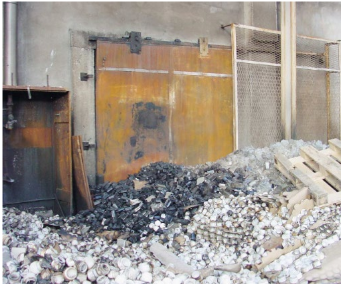
After the fire, on one side of a fire door ...
