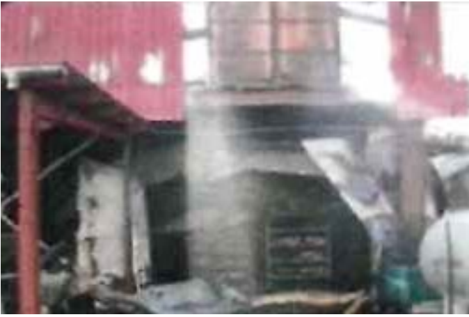
↑ Gas tank, intact amid the rubble
