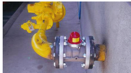
Seismic shutoff valve for natural gas line
