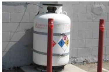
Flammable liquid tank strapped to wall
