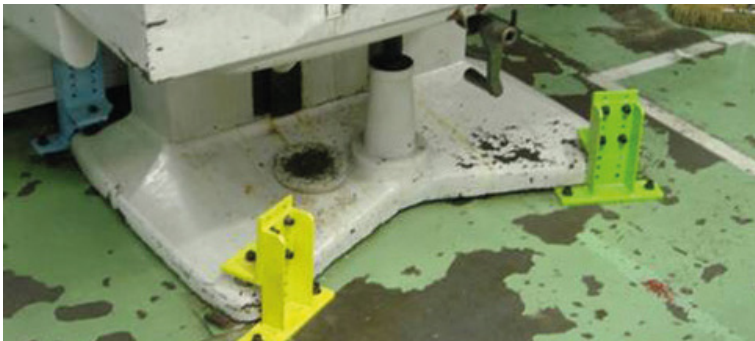
Production equipment anchored to the floor
