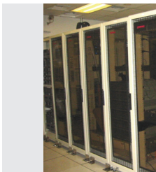
Computer server racks anchored to the floor
