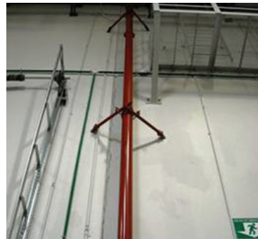
Sprinkler riser with sway bracing
