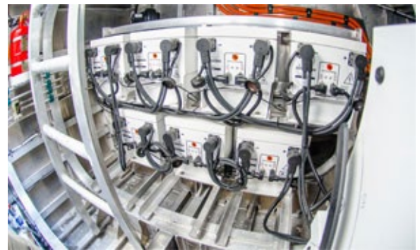
Lithium-ion batteries in a rack on a marine vessel.
