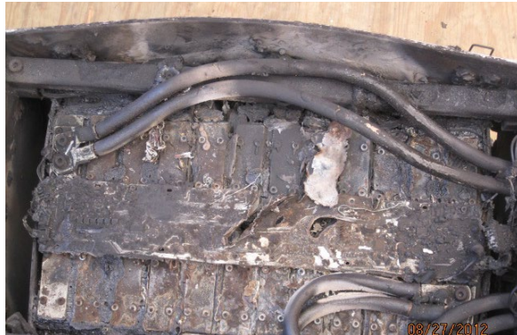
Burned out lithium-ion battery
