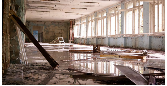
Water damage to building under construction
