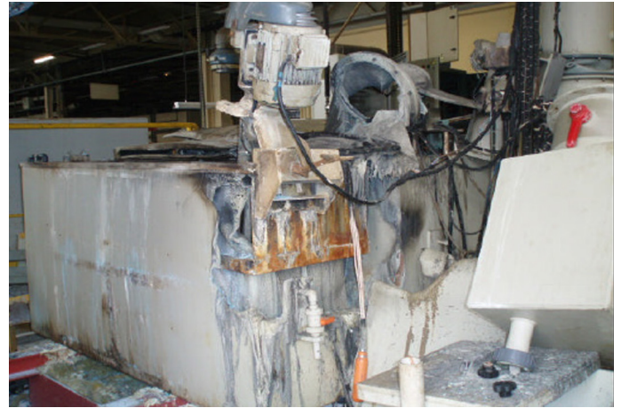
Fire Damage to Plastic Tank
