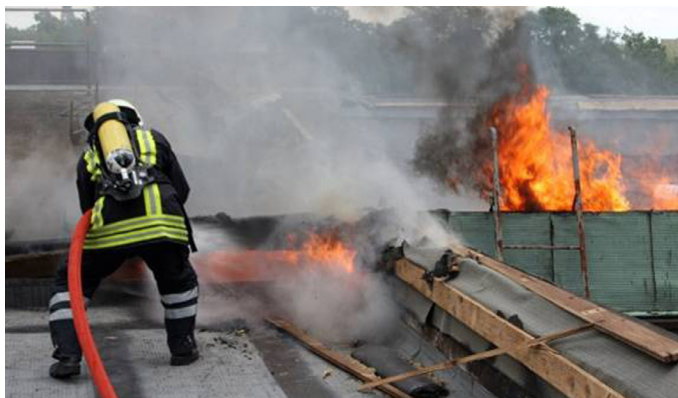
Fire caused by roofing operations
