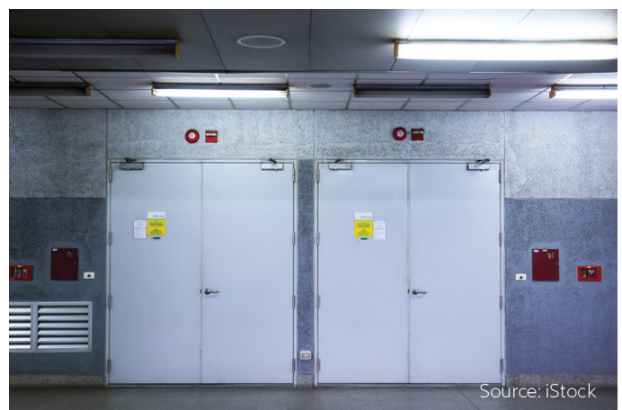
Only authorized personnel should be allowed access to the refrigerated storage area.
