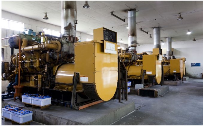
Diesel Engine Driven Emergency Generators
