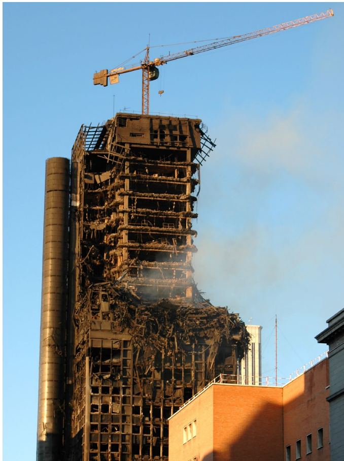
The burnt building Windsor Tower in Madrid, Spain on February 13, 2005
