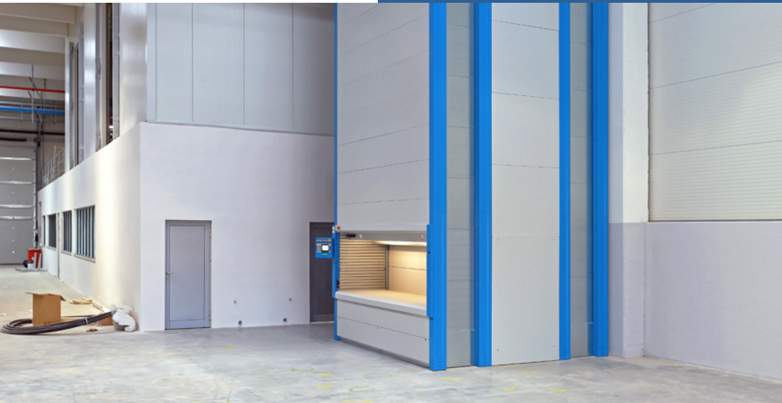
Vertical automated storage system (VASS) installed in a warehouse
