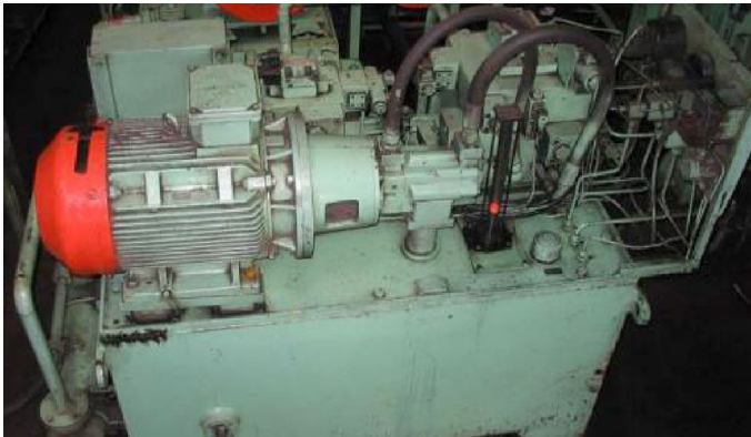
Hydraulic system with motor, pump and valves
