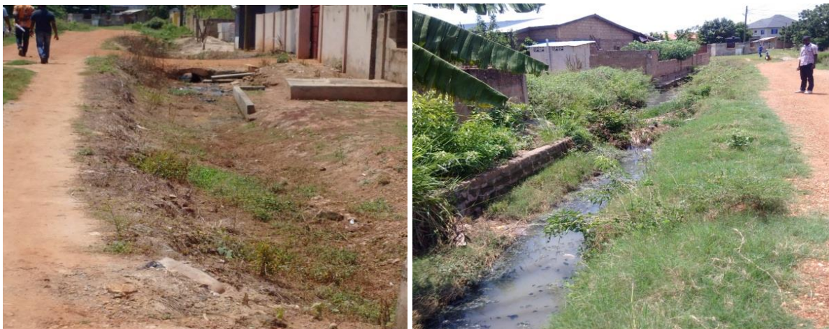
Figure 35: Examples of poorly constructed and maintained drainage systems in GAMA (Adentan). Source: (Annan, Adarkwah, Mattah, & Awuni, 2019).
