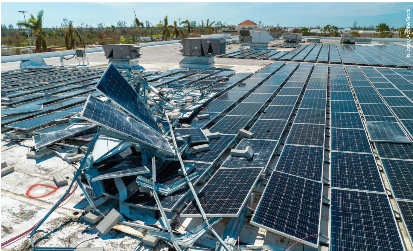
Roof-mounted equipment, such as solar panels, is particularly vulnerable when storms hit
