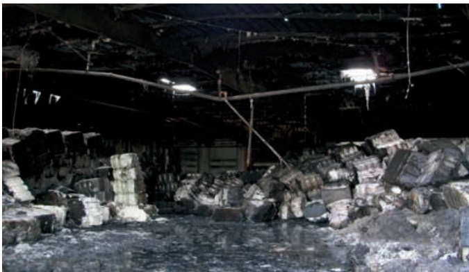
The result of a warehouse with an inadequately designed sprinkler system
