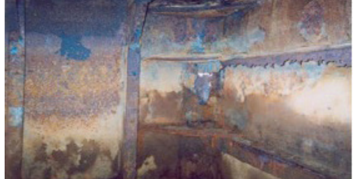
Heavy wastage and deterioration of internal structural members
