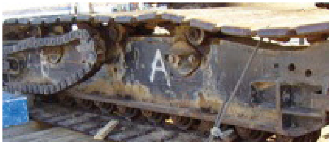
Insufficient securing. Only one (1) \frac{3}{4} " wire looped over treads at each end. Crane mats are not secured to the deck.
